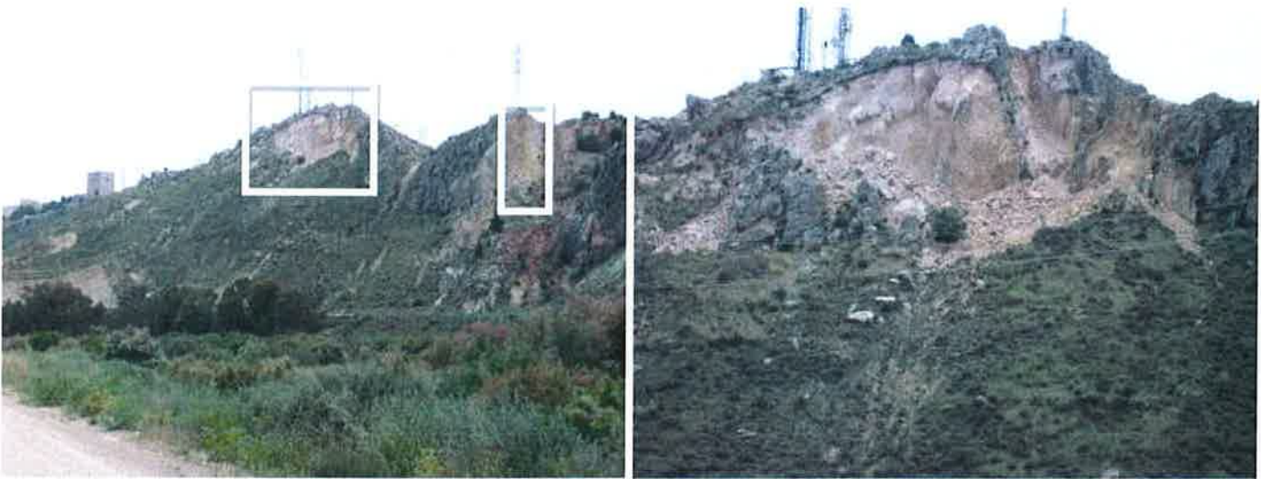
Figure 4.4.1a: Rock-falls and debris on the summit of the north slopes of the Pantano de Puentes road. Their attribution to the earthquake is presumed. The westernmost one (on the right on the first photo) corresponds in part with a previous instability.
