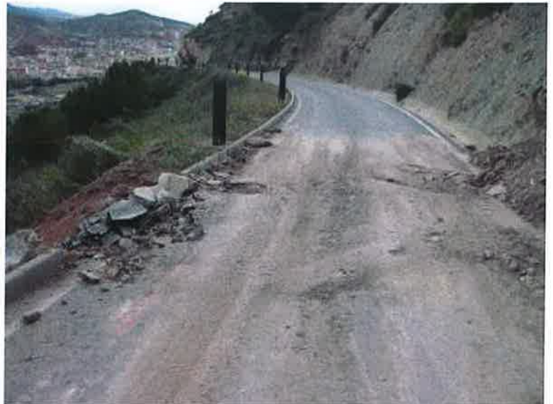
Figure 4.2.4b: Damage on the pavement of the up-the-hill road to the castle due to the fall and rebound of the block shown in figure 1.4a.
