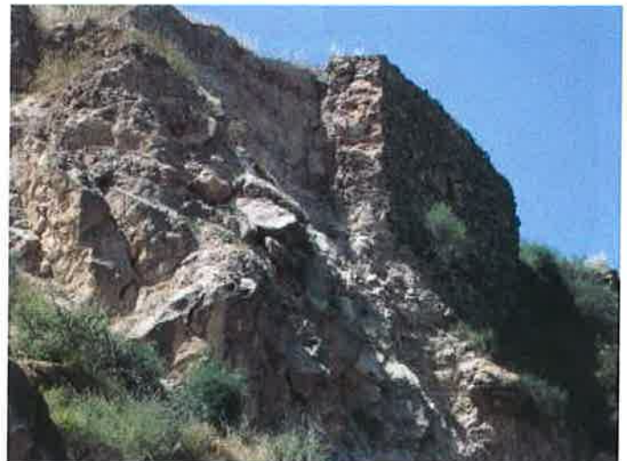
Figure 4.2.1f: Close up of the fall of part of an old retaining wall. It can be observed that the intrados filling remains meta-stable. This type of instability also appears on the south face of Lorca's castle cliff (see figure 2.1).
