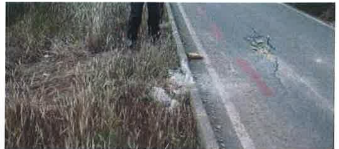
Figura 4.2.1d: Moderate damage on the down-the-hill road caused by the rebound of the block detached from the easternmost point of the cliff (figure 1.b).
