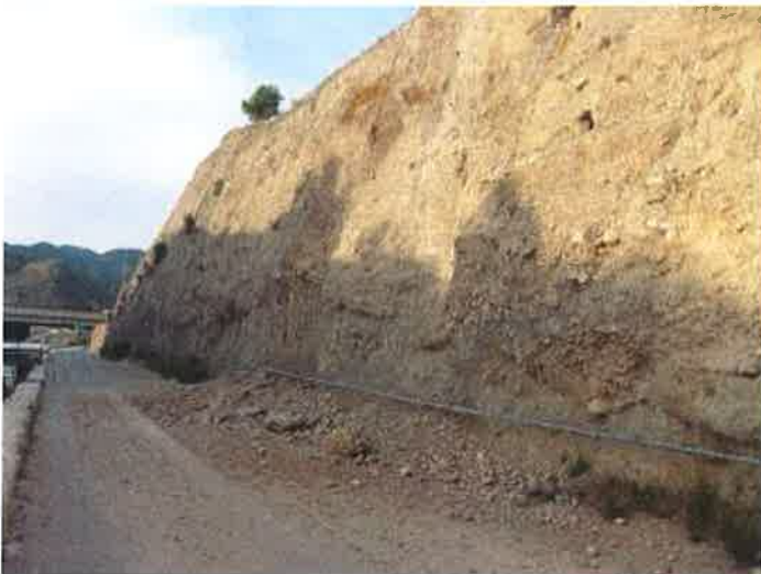
Figure 4.9: Shallow debris falls attributed to the May earthquakes on a service road of the Tajo-Segura canal.
