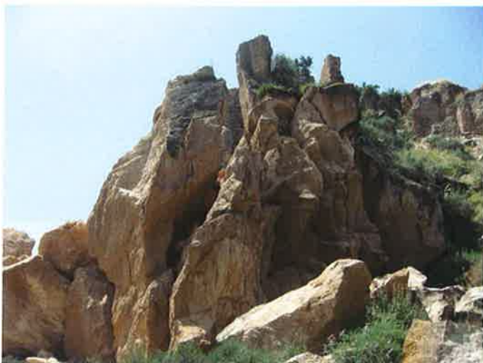
Figure 4.2.1e: Close-up of the collapse of the easternmost point of the castle cliff (looking South) and of the general conditions of the rock mass at this site. On the upper right corner it is observed part of a fallen wall (see figure 1.1f).
