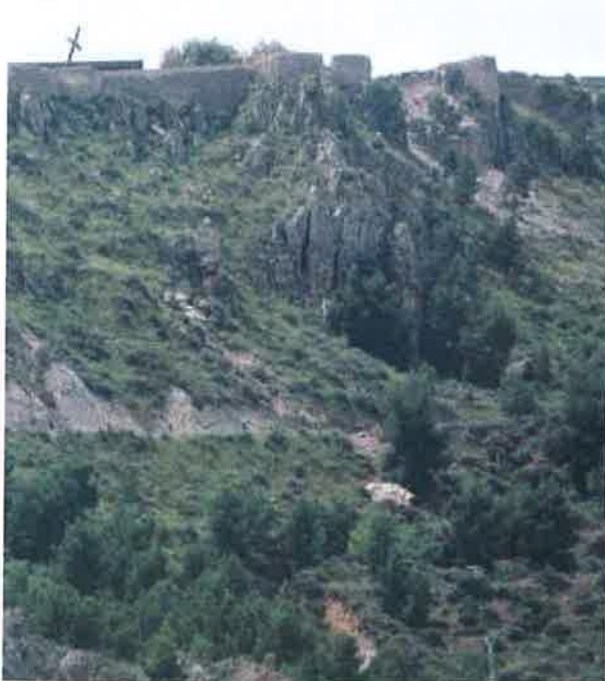
Figure 4.2.4a: Rock-fall of metric size that damaged badly the road (see figure 1.4b).
