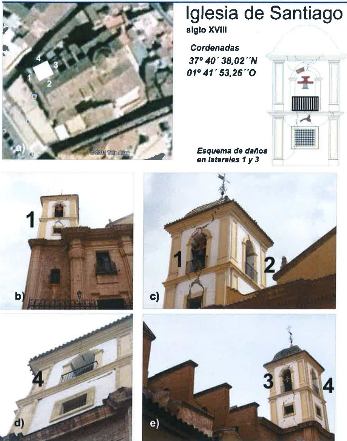
Figure 5.3: Damage in the church's tower of Santiago.
