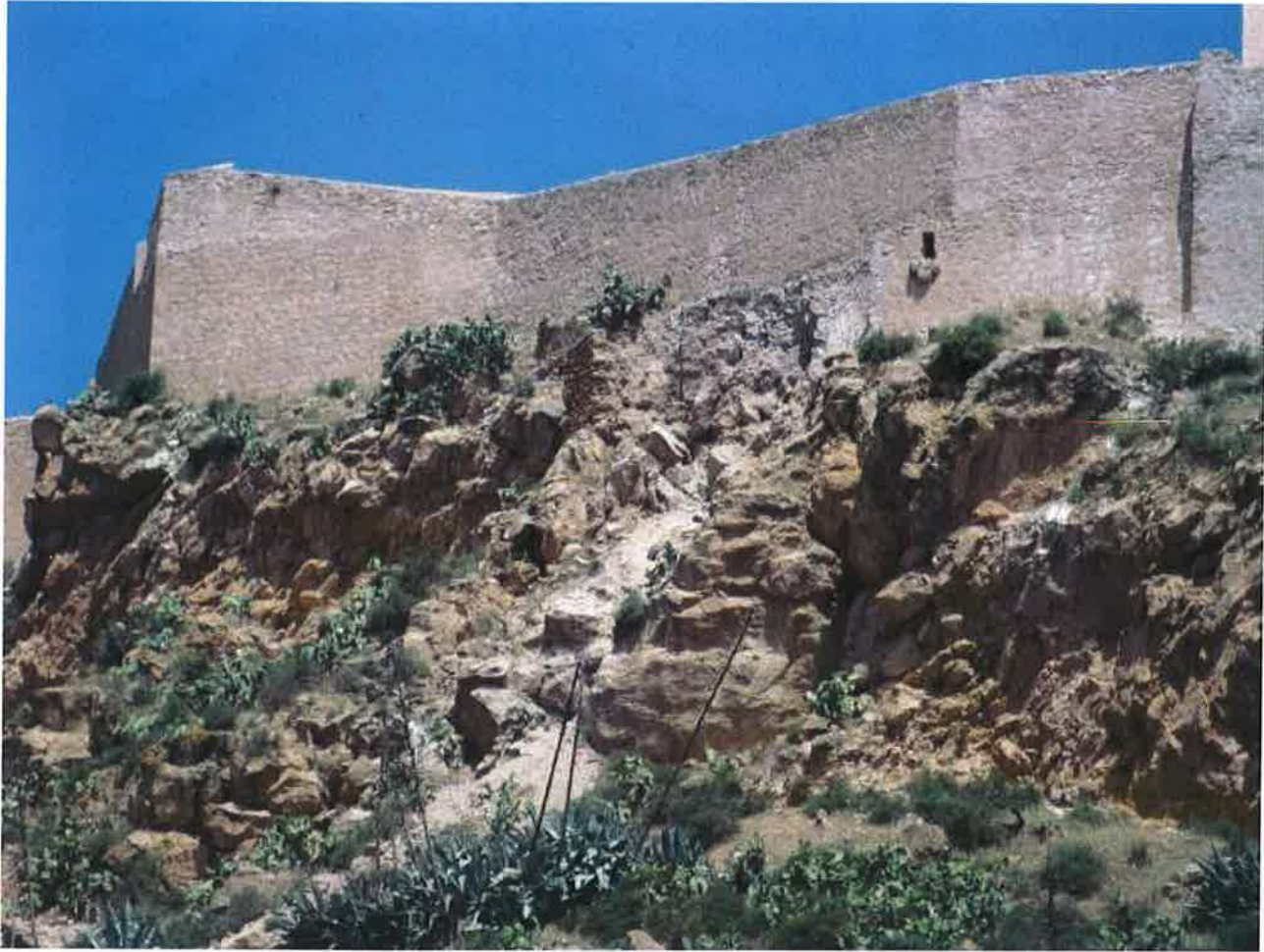
Figura 4.3.1: Collapse of an old retaining wall attached to the external wall of the Lorca's castle on its south face. This instability warned the dwellers of the houses situated right under the cliff, which asked us whether it was safe to return back to their places.
