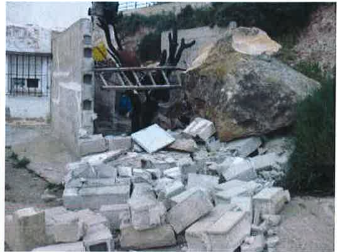
Figure 4.2.1c: Result of the impact on a wall made of concrete blocks enclosing the patio of a house from a rock detached from the easternmost point of the cliff.
